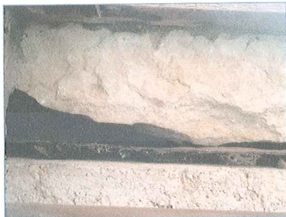
Photo 5. Crevice above gable window
