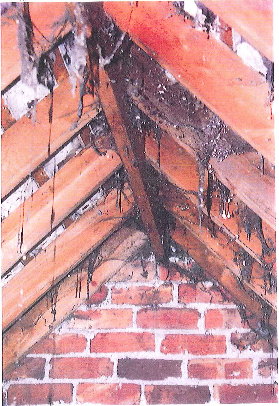
Appendix 5: Photo taken looking East in the loft of the School Room.
