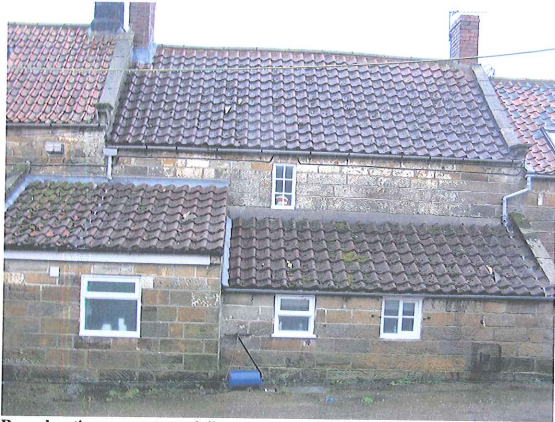
Rear elevation, concrete roof tiles to centre two storey section and both single storey lean-to sections. Clay pantiles to upper roofs on either side of main structure.
