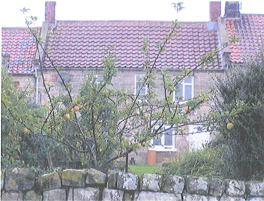
Front elevation, concrete tiles on centre roof slope, clay pantiles to roofs either side.
