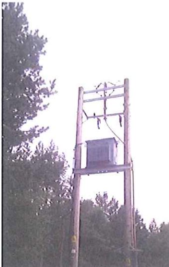
Existing Transformer pole mounted at the entry to the site
