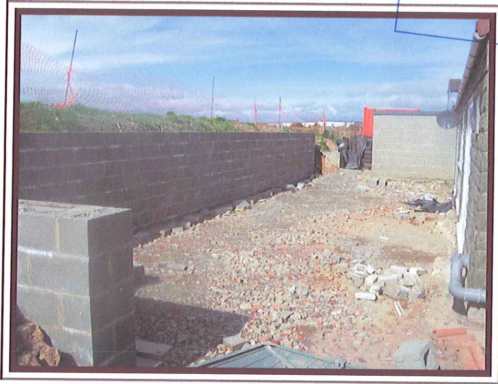
View of retaining wall on the western element of the sun terrace/patio
