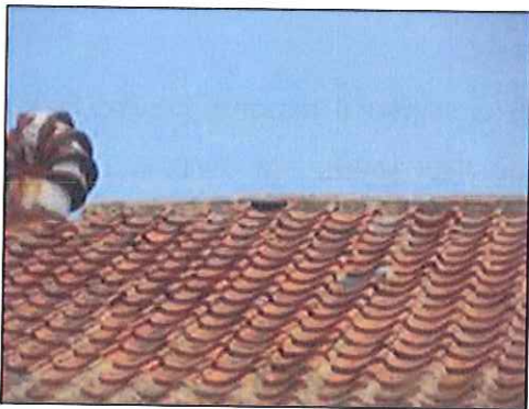
Photo 5: Gap along ridge
