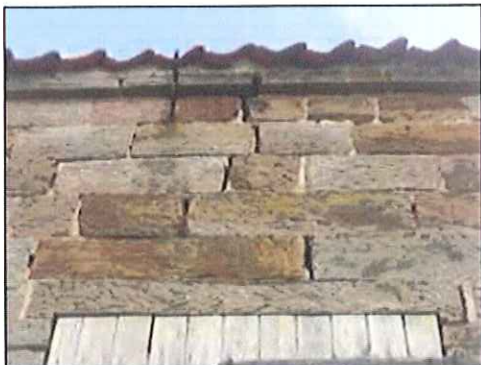
Photo 3: External masonry crevices
