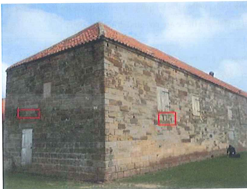
Photo 6: Emergence locations at northwest corner of building
