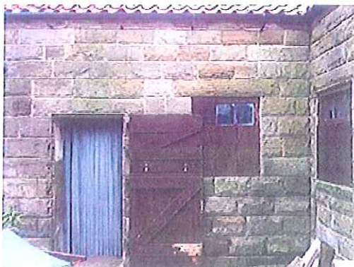
Rear elevation: Damaged and boarded up windows
