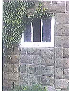
Road side elevation: Unsightly stone infill to former door.
