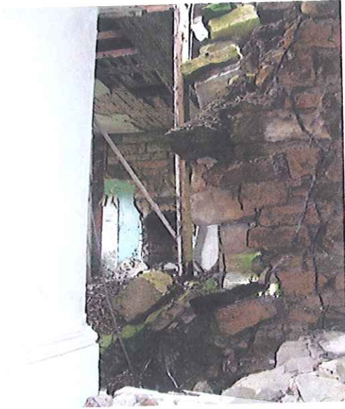
Landing through to Rear Bedroom Collapsed Floor / Wall
