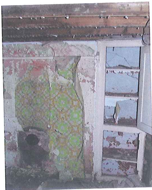
Kitchen Boiler Position Side Wall Cupboard
