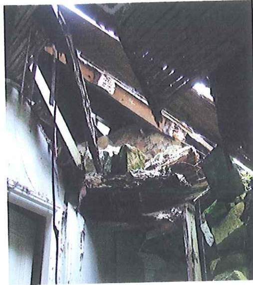
Landing - collapsed Ceiling / Roof
