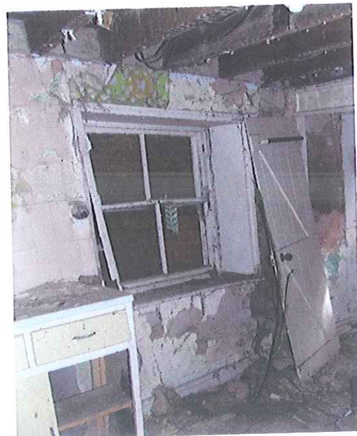
Kitchen - Ceiling Boards Collapsed
