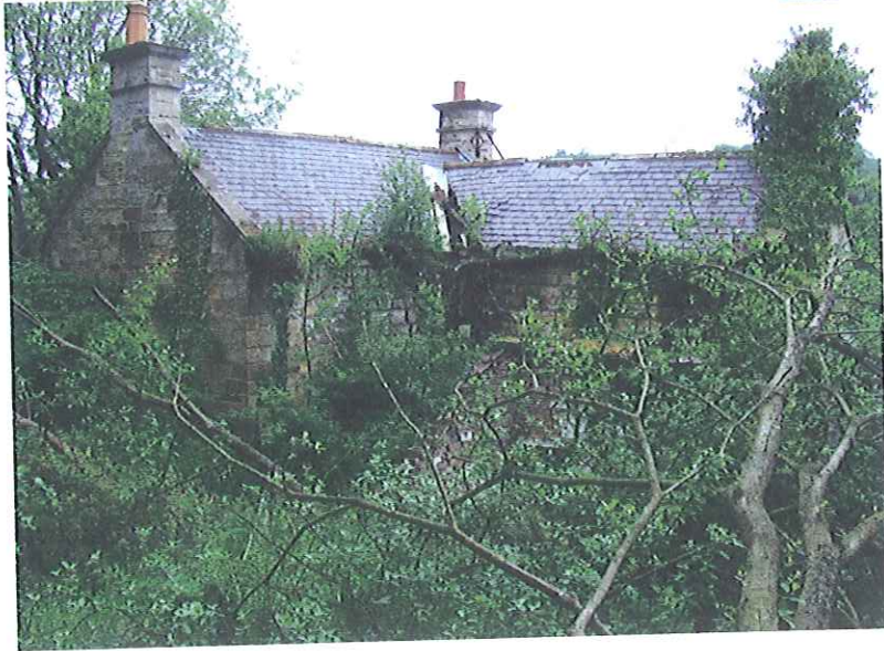
Collapsed Wall / Roof at junction of extension and Main Structure
