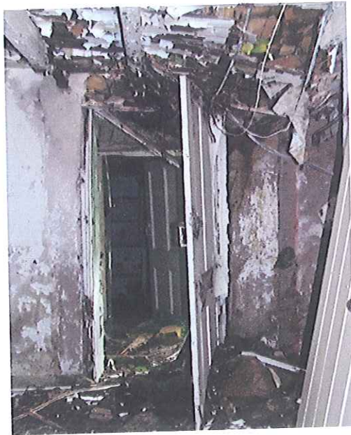
From North Room through Rear Lobby to Extension Kitchen with 4 Panel Door
