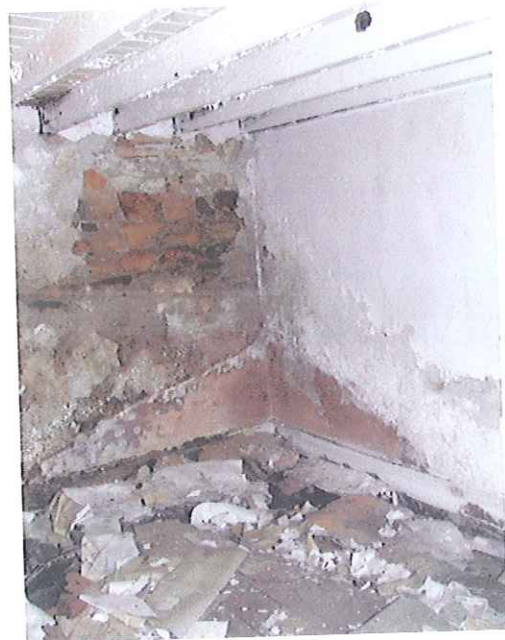
Collapsed Timber Floor
