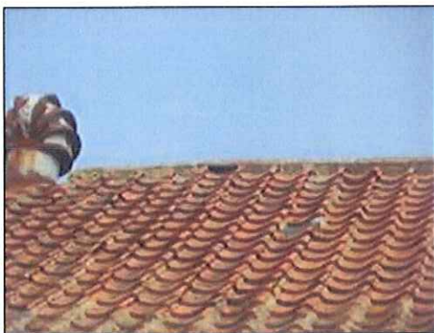
Photo 5: Gap along ridge
