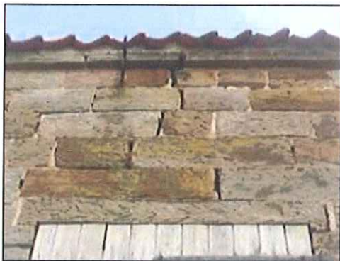
Photo 3: External masonry crevices
