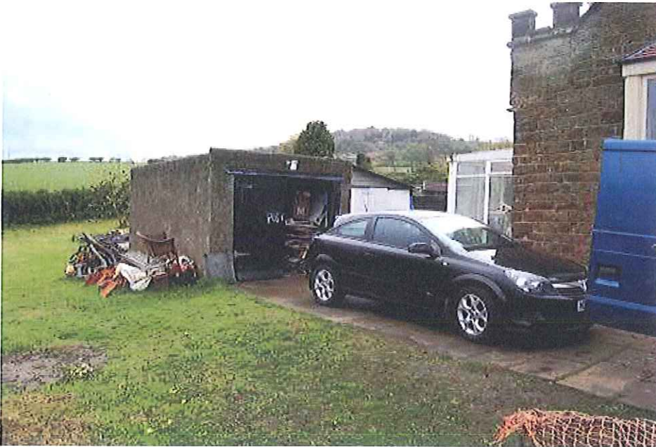
The existing structures are of poor material construction and poorly sited in relation to the main residence.
