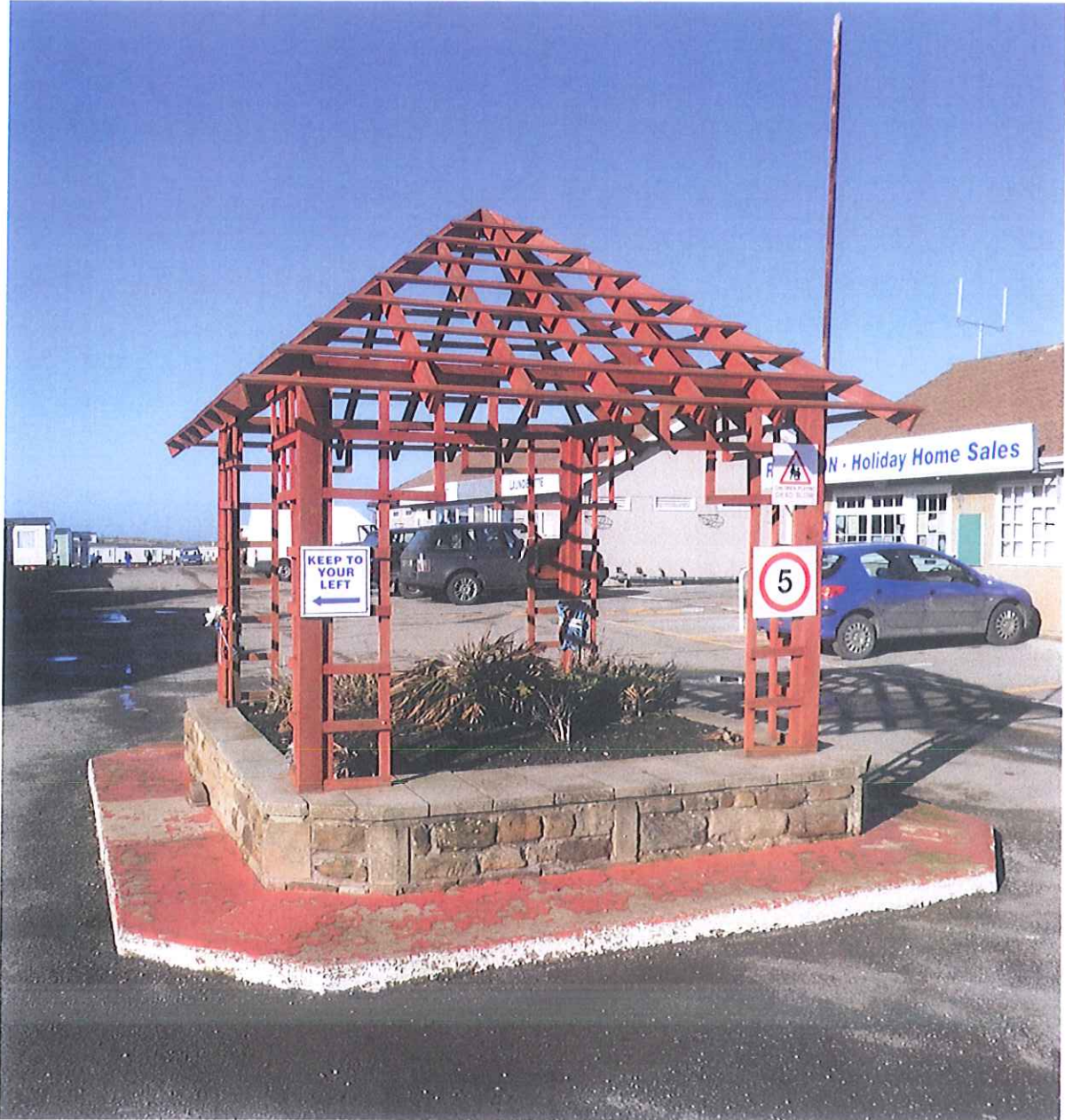
Figure 17. The existing structure proposed for replacement is illustrated below
