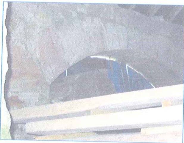
Figure 5 Gaps in wooden doors with daylight visible (internal).
