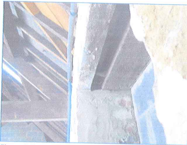
Figure 4 Gap in wooden lintel above block up doorway.
