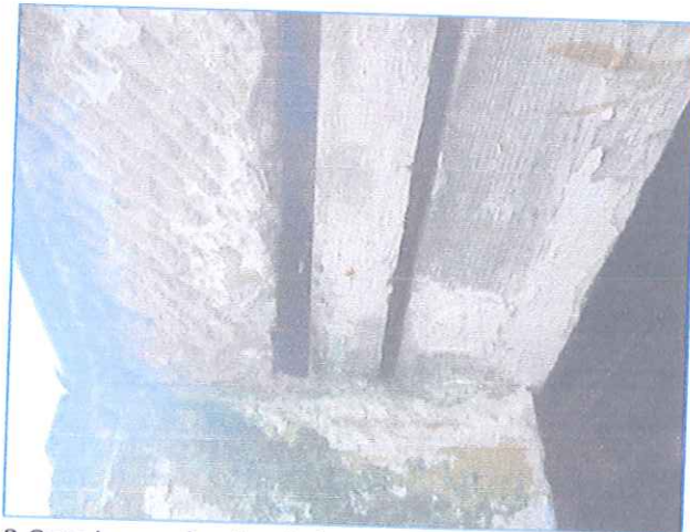
Figure 2 Gaps in wooden lintel above main entrance (east elevation).
