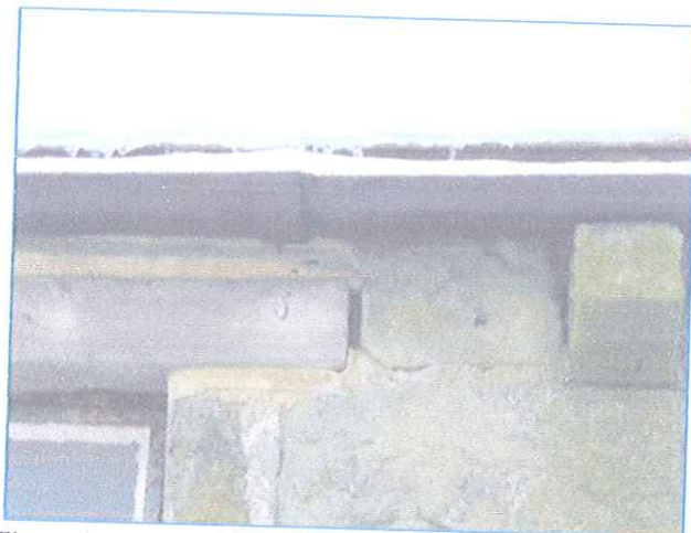
Figure 3 Gap in stone work and wooden lintel (external).
