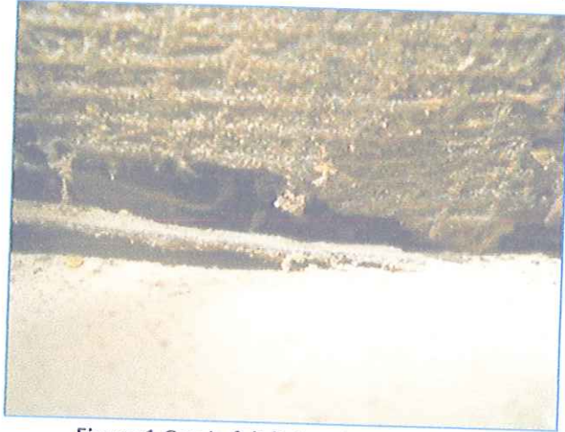
Figure 1 Gap in felt lining above wall top.
