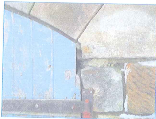
Figure 6 Gaps in wooden doors (external).
