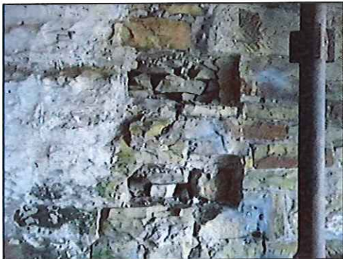
Photo 7: Crevices within stone wall
