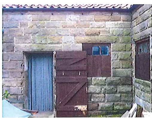
Rear elevation: Damaged and boarded up windows
