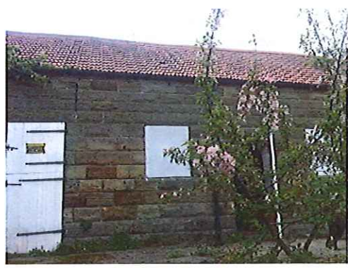
Road side elevation: Windows boarded up
