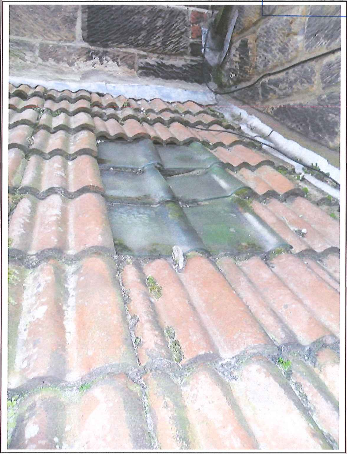
Photo 4 Roof slope to extension in June 2013 prior to works. Note damaged glass tiles.
