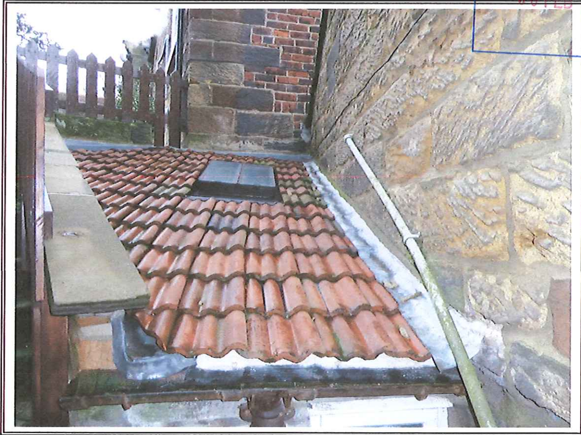
Photo 5 Roof after completion of works. Note same roof pitch and re-used tiles.
