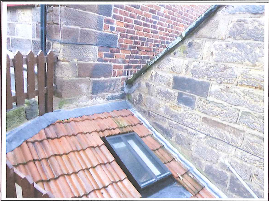
Photo 6 Roof after completion of works. Note conservation rooflight in position of glass tiles.
