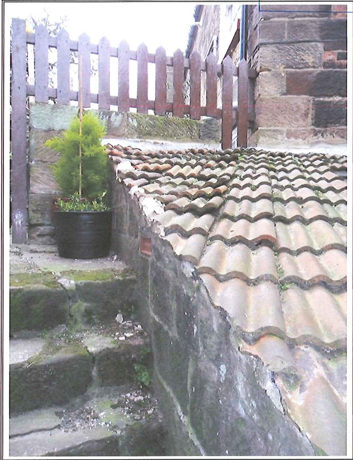
Photo 3 Roof slope to extension in June 2013 prior to works. Note damaged tiles.
