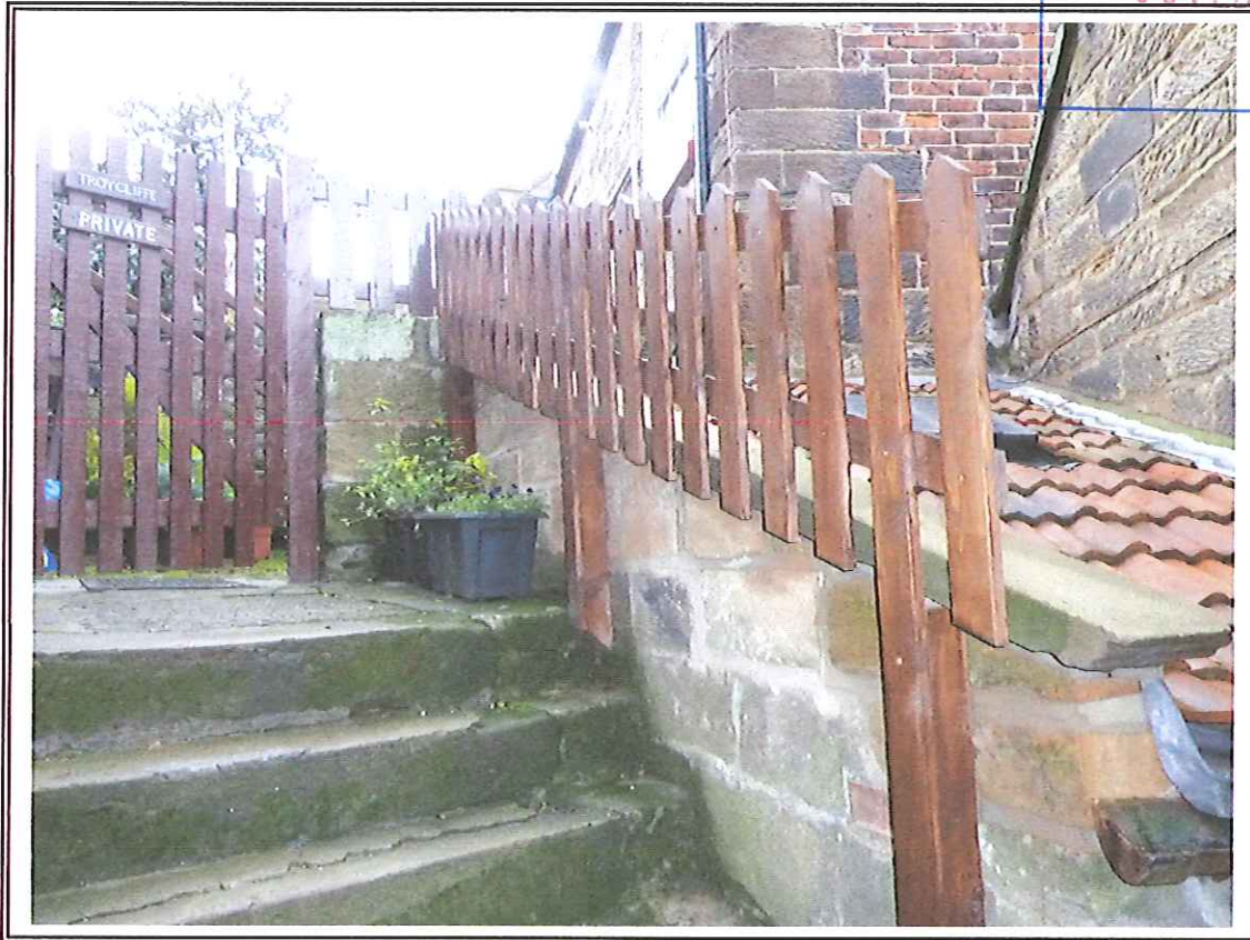
Photo 7 Edge of roof after completion of works. Note picket fence to match existing yard fence.
