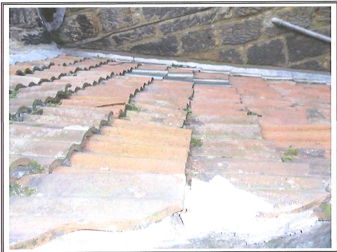
Photo 2 Roof slope to extension in June 2013 prior to works. Note damaged tiles.
