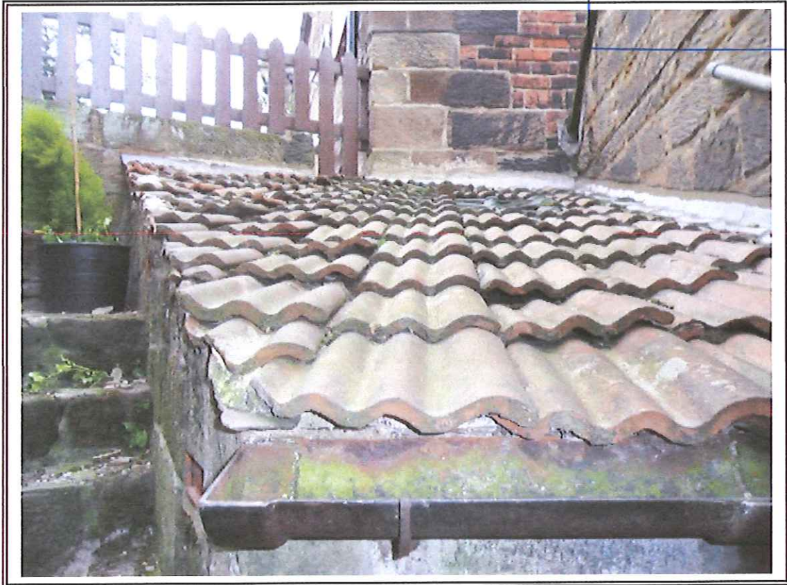
Photo 1 Roof slope to extension in June 2013 prior to works. Note damaged tiles.
