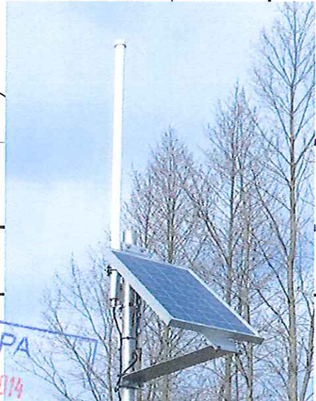
1m vertical antenna attached to 30cm J-Mount bracket 1m vertical and 3cm diameter on north elevation
