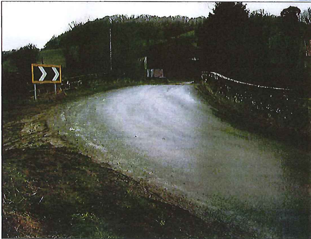
Photograph 1: View across bridge from south. Note narrow carriageway width at centre of bridge (4.6m approx.) and poor alignment.
