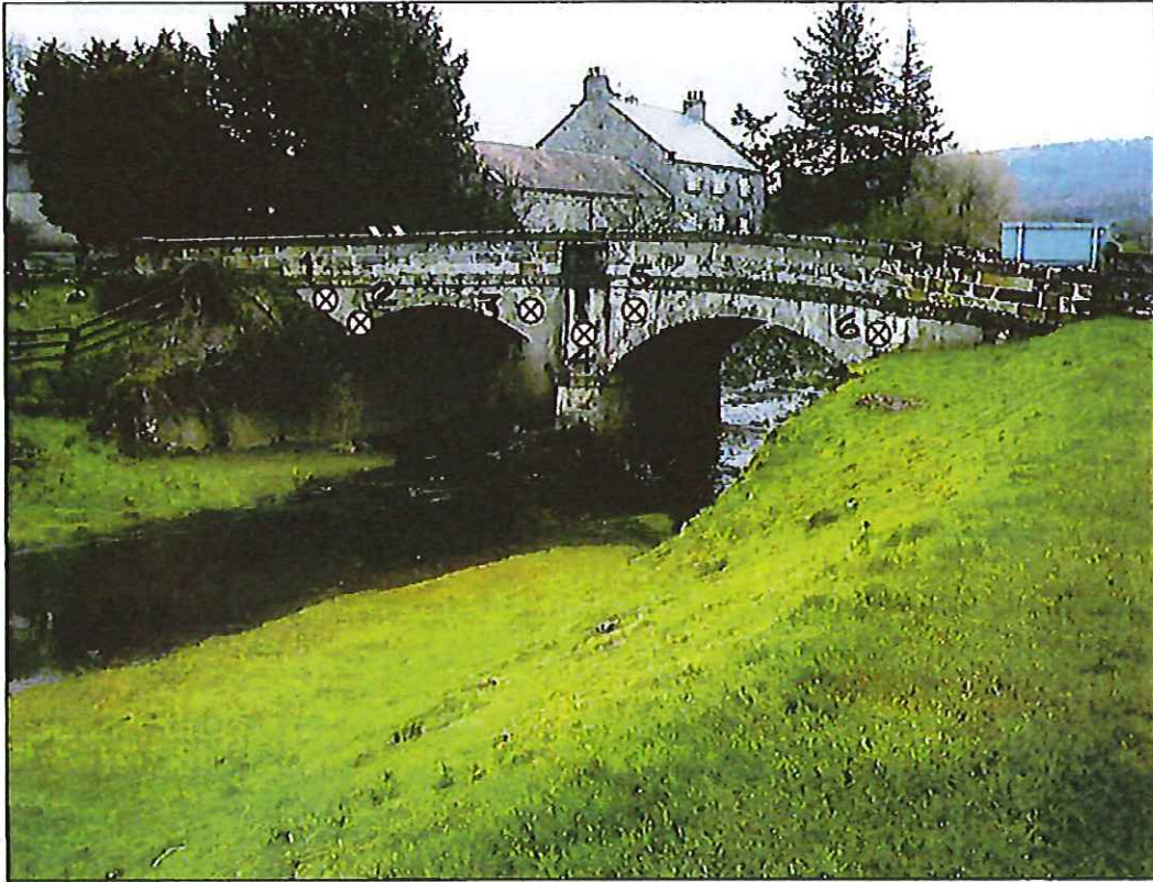
Photograph 3: West upstream elevation. Vegetation clearance from NW corner and from pier. Cores required in indicative locations as shown.
