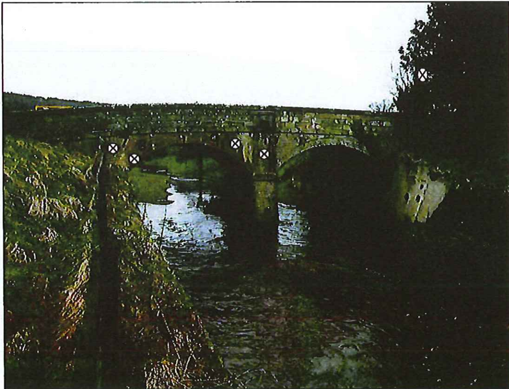
Photograph 4: East downstream elevation. Vegetation clearance required from NE corner. Cores required in indicative locations as shown.
