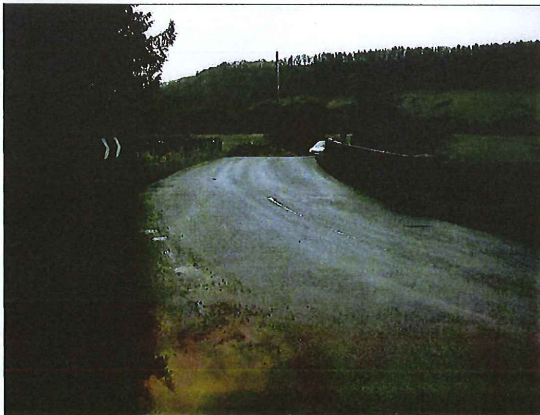
Photograph 2: View across bridge from north. Note narrow carriageway width at centre of bridge (4.6m approx.) and poor alignment.
