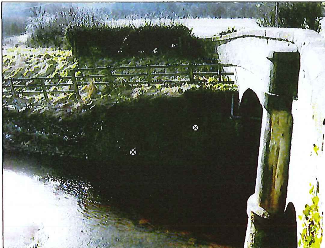
Photograph 8: South east wing wall. Cores required in indicative locations as shown.
