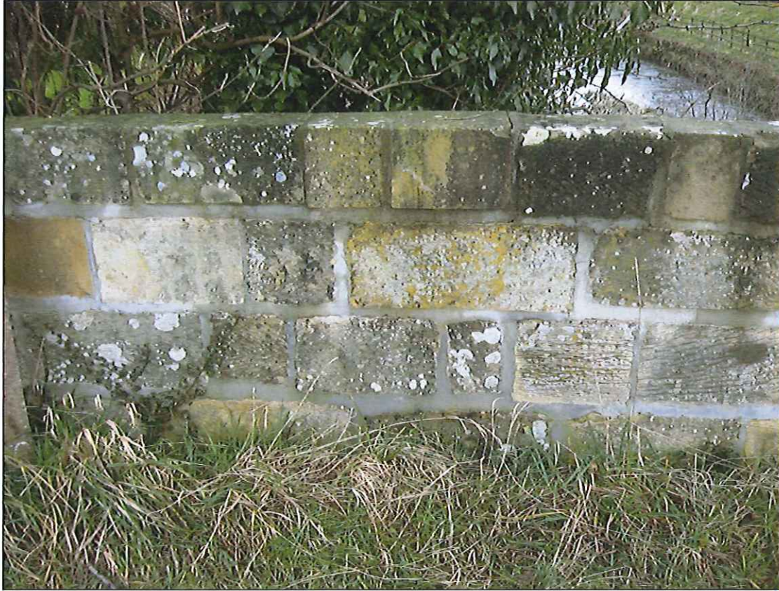
Photograph 39: Repaired area of parapet at north east corner of bridge.
