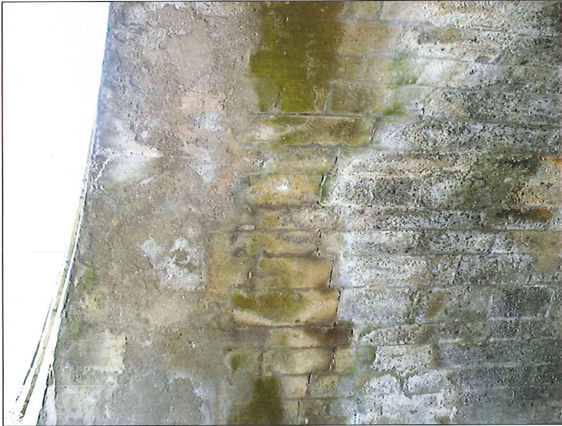
Photograph 31: Concrete widening #3 to western upstream side of north span. Note circumferential cracking in masonry further into arch.
