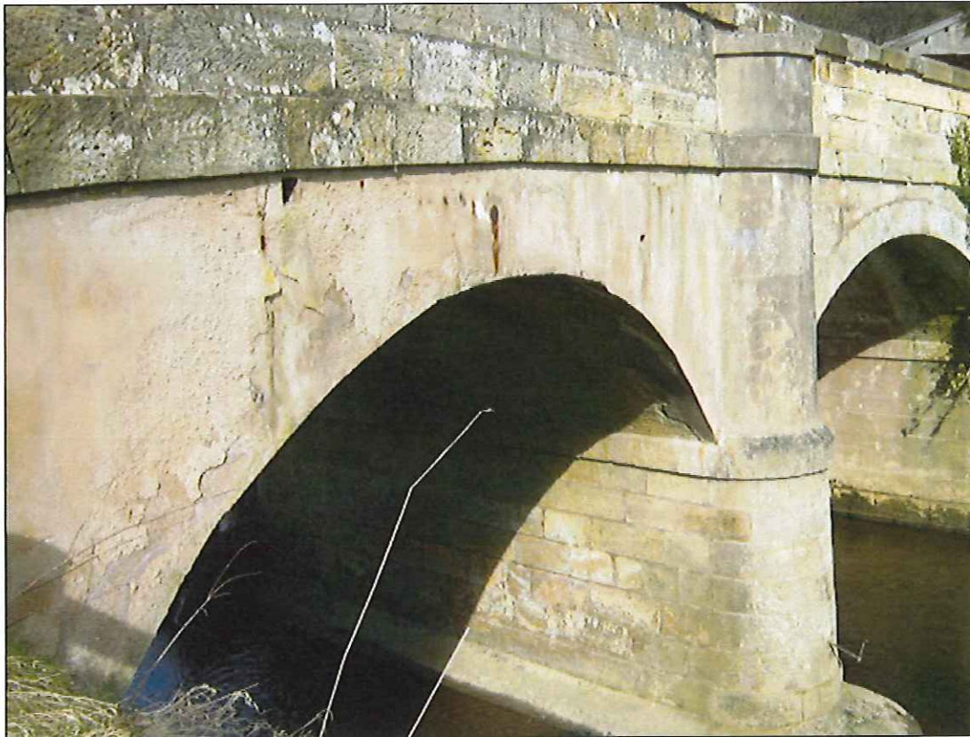
Photograph 11: Eastern downstream elevation southern span with rendered mass concrete arch widening and spandrel walls.
