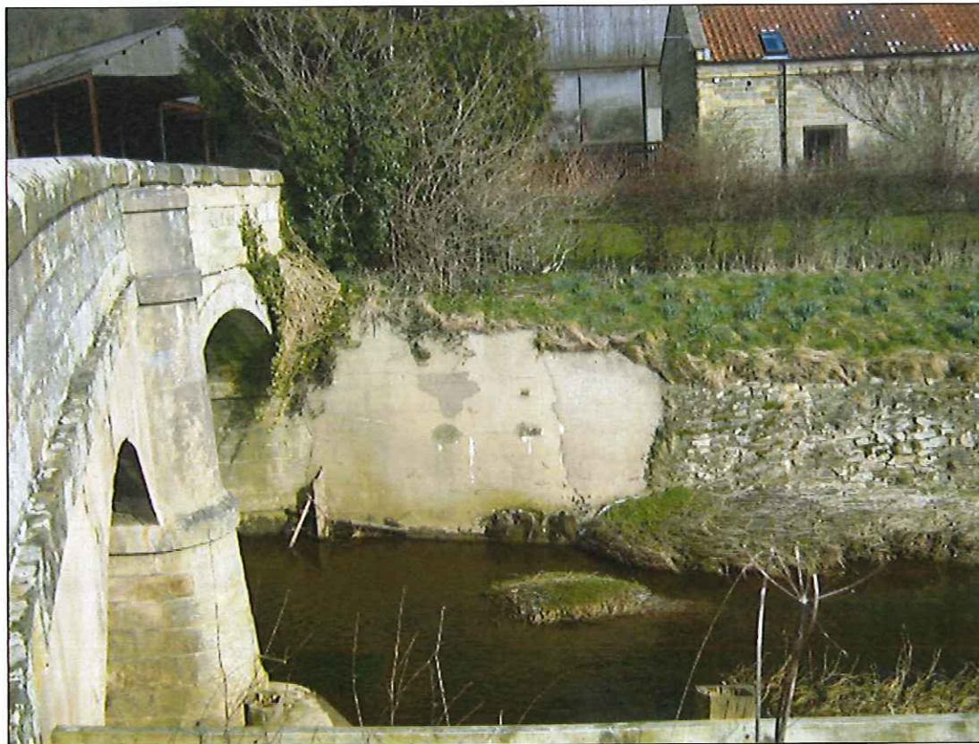
Photograph 20: North east wing wall constructed of mass concrete with thin rendering to face.
