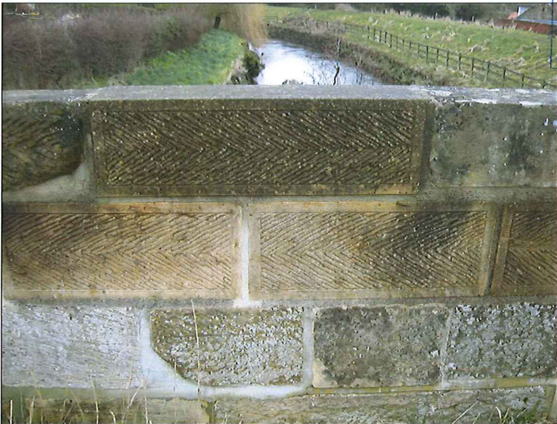
Photograph 40: Repaired area to eastern downstream parapet showing herringbone tooling to replicate original stone.
