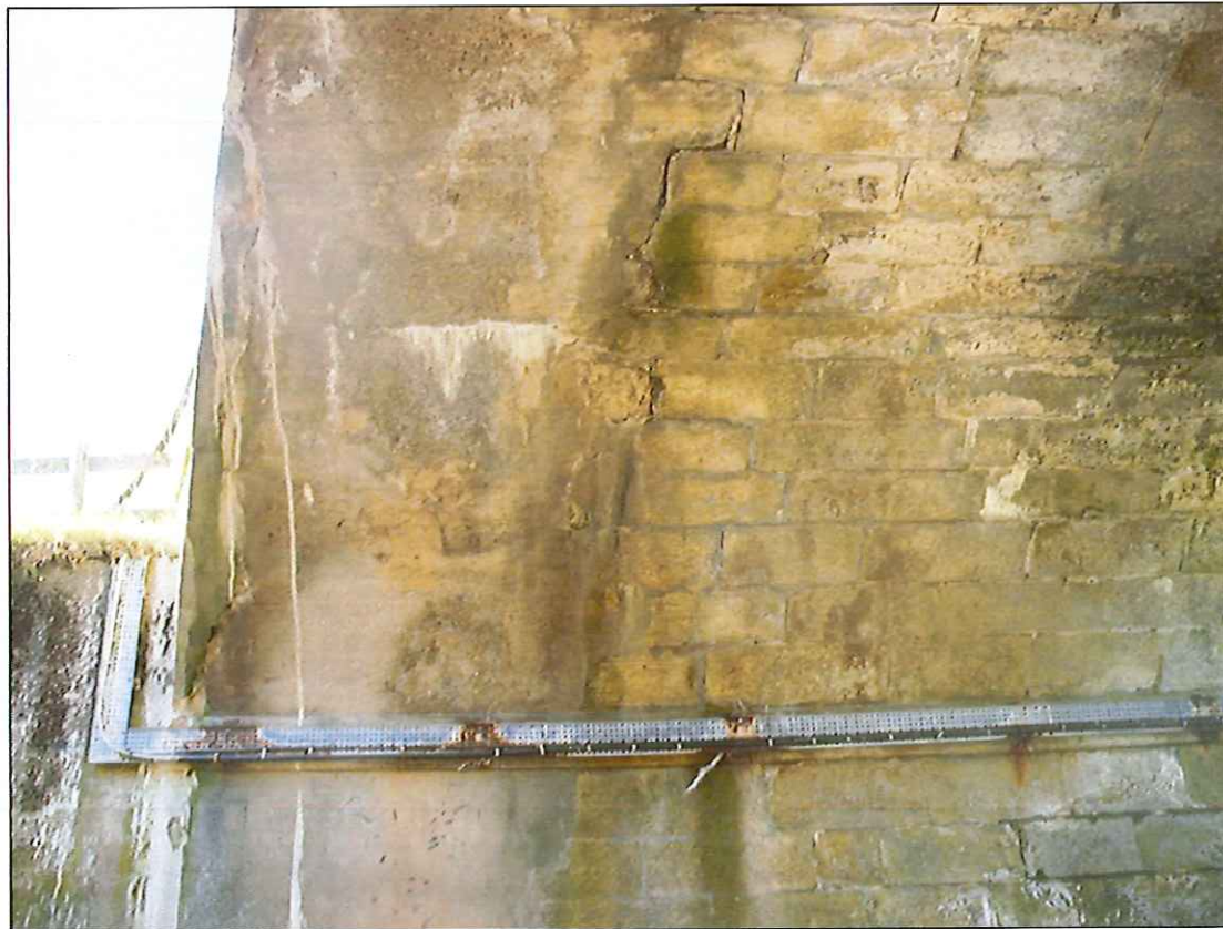
Photograph 24: Concrete widening #2 to eastern downstream side of south span. Note circumferential cracking.
