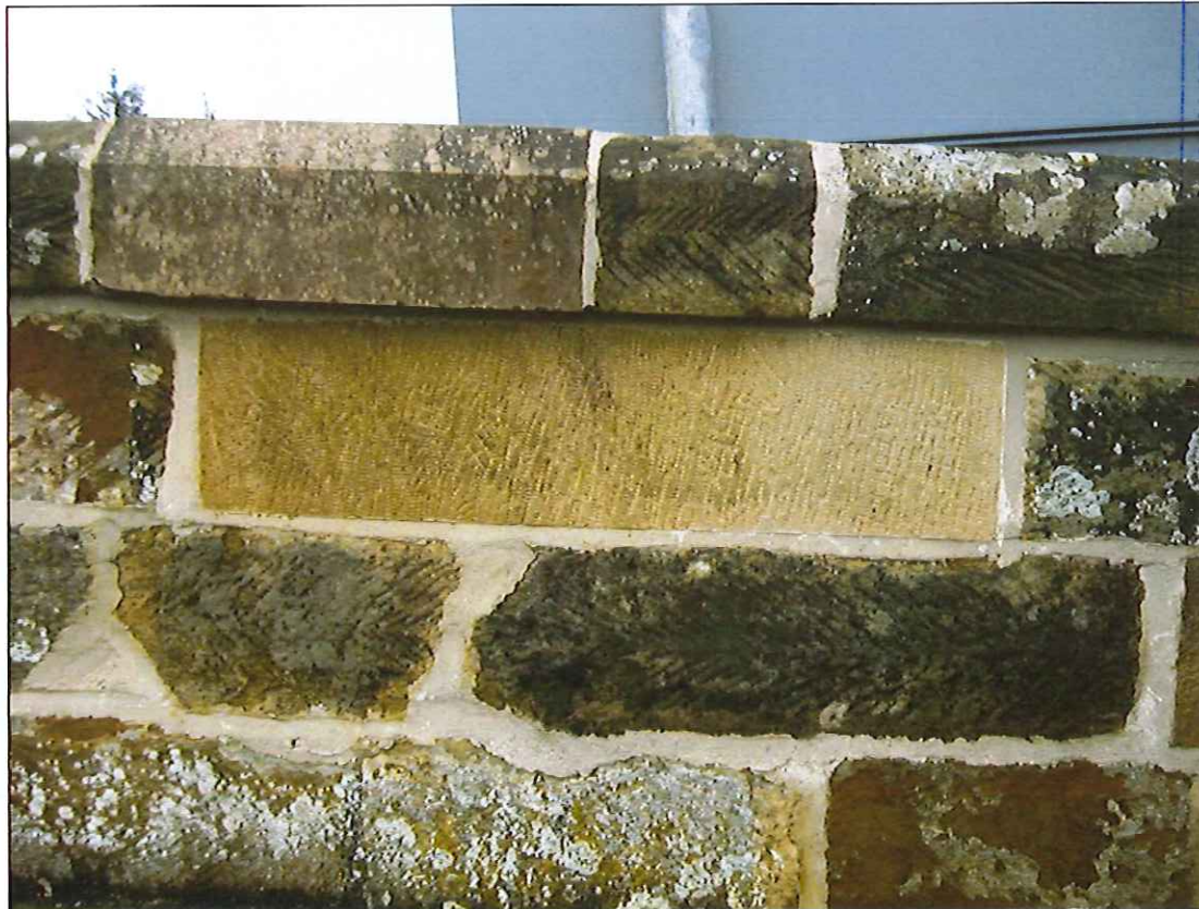
Photograph 36: Outside face of parapet near south west corner of bridge showing replacement stone with incompatible tooling.
