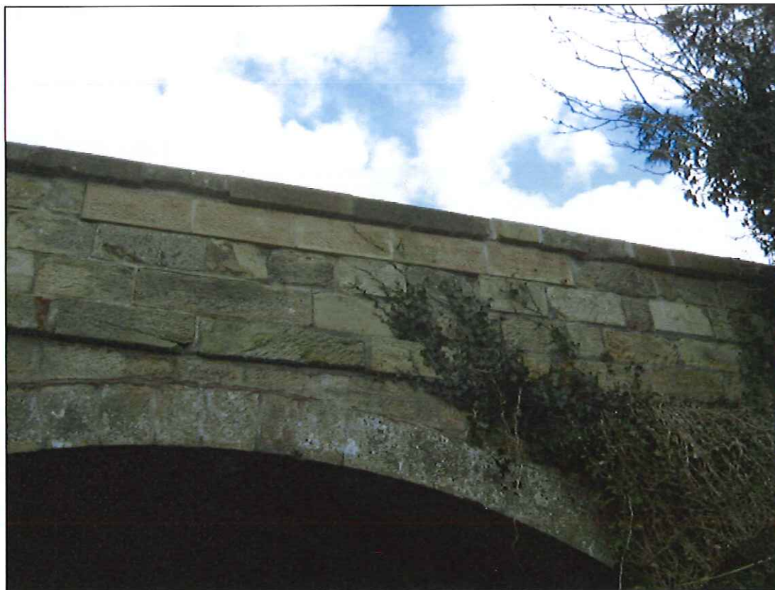
Photograph 12: East downstream elevation northern span with original masonry arch and spandrel walls remaining. Note repairs to parapet.
