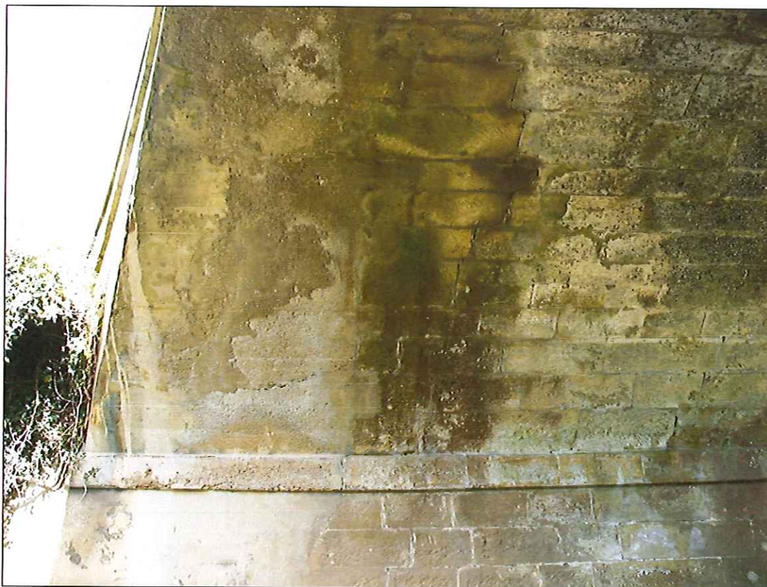
Photograph 30: Concrete widening #2 to western upstream side of north span. Note circumferential cracking in masonry further into arch.
