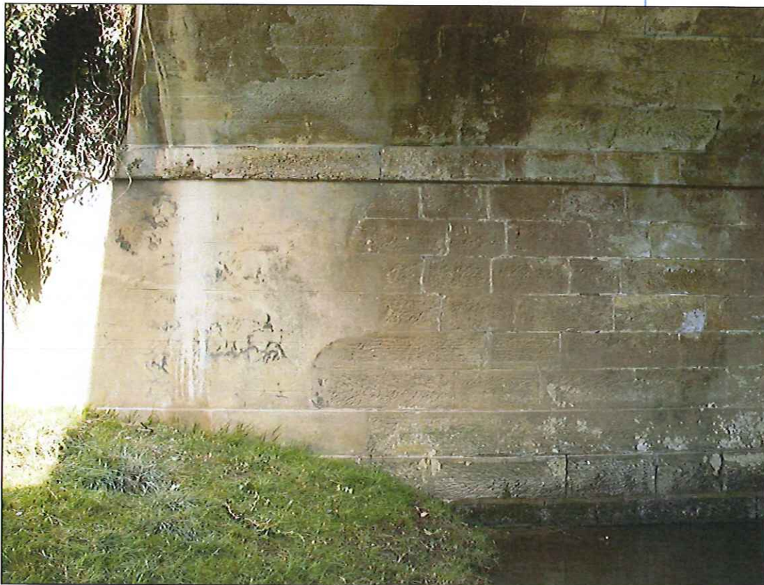
Photograph 29: Concrete widening #1 to western upstream side of north span at north abutment.
