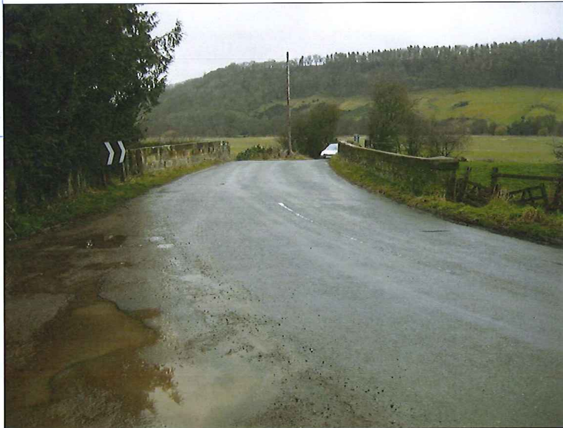
Photograph 4: View across bridge from north. Note narrowing width between parapets and poor forward visibility.
