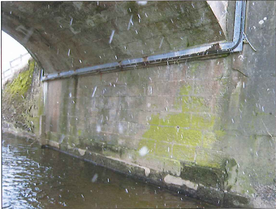
Photograph 15: South abutment. Mass concrete widened section to south east corner of bridge to left of picture.
