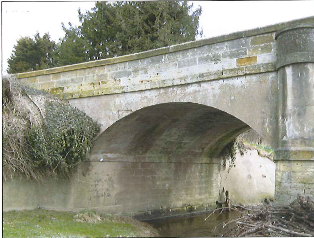
Photograph 19: North abutment. Widened mass concrete section of abutment is at left hand end of arch in picture.
