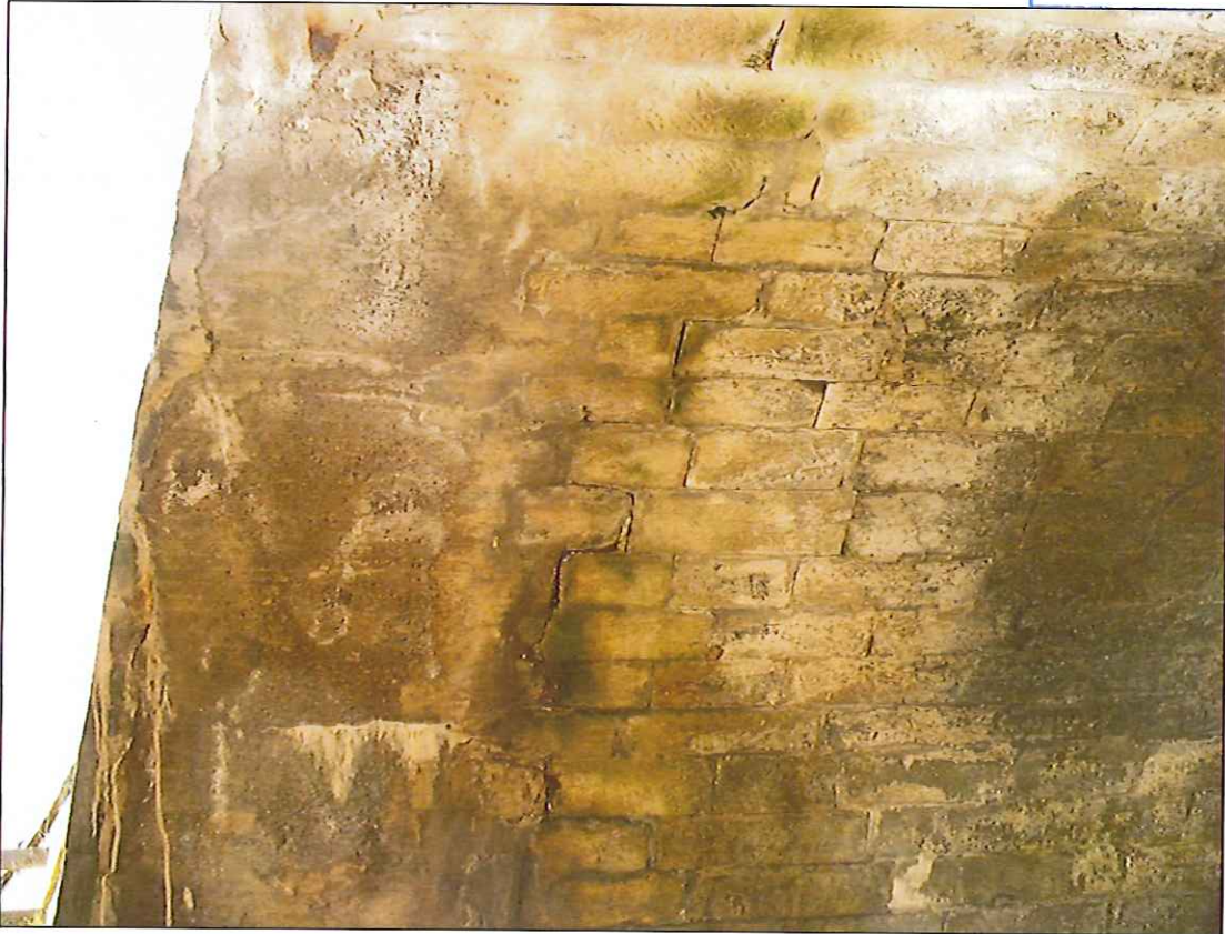
Photograph 25: Concrete widening #3 to eastern downstream side of south span. Note extensive circumferential cracking.
