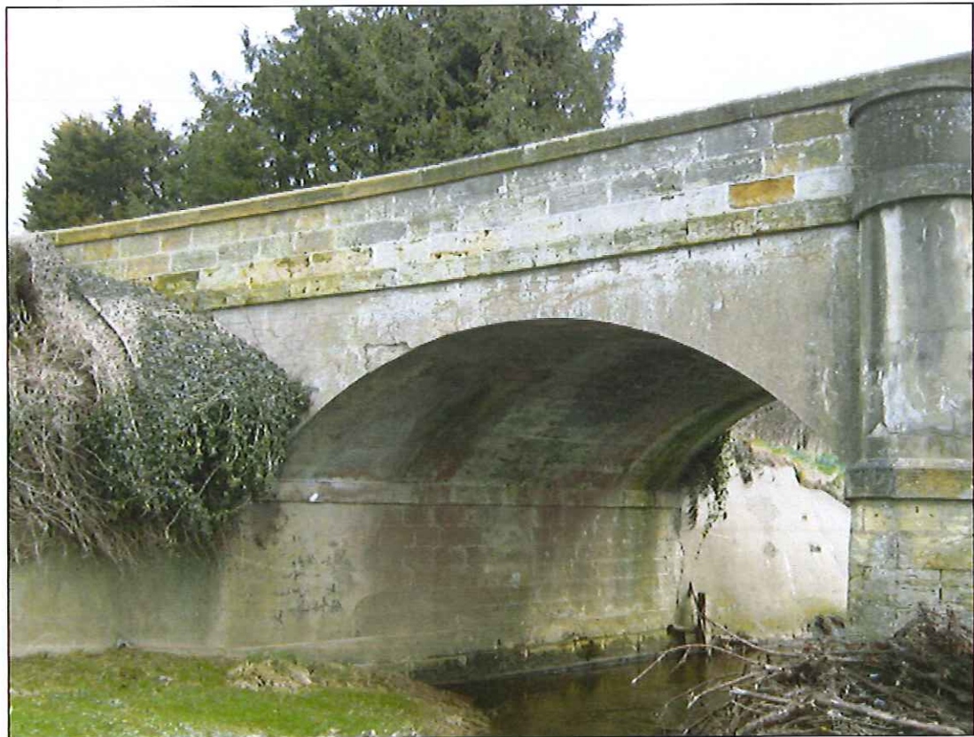
Photograph 8: West upstream elevation northern span with rendered mass concrete arch widening and spandrel walls.
