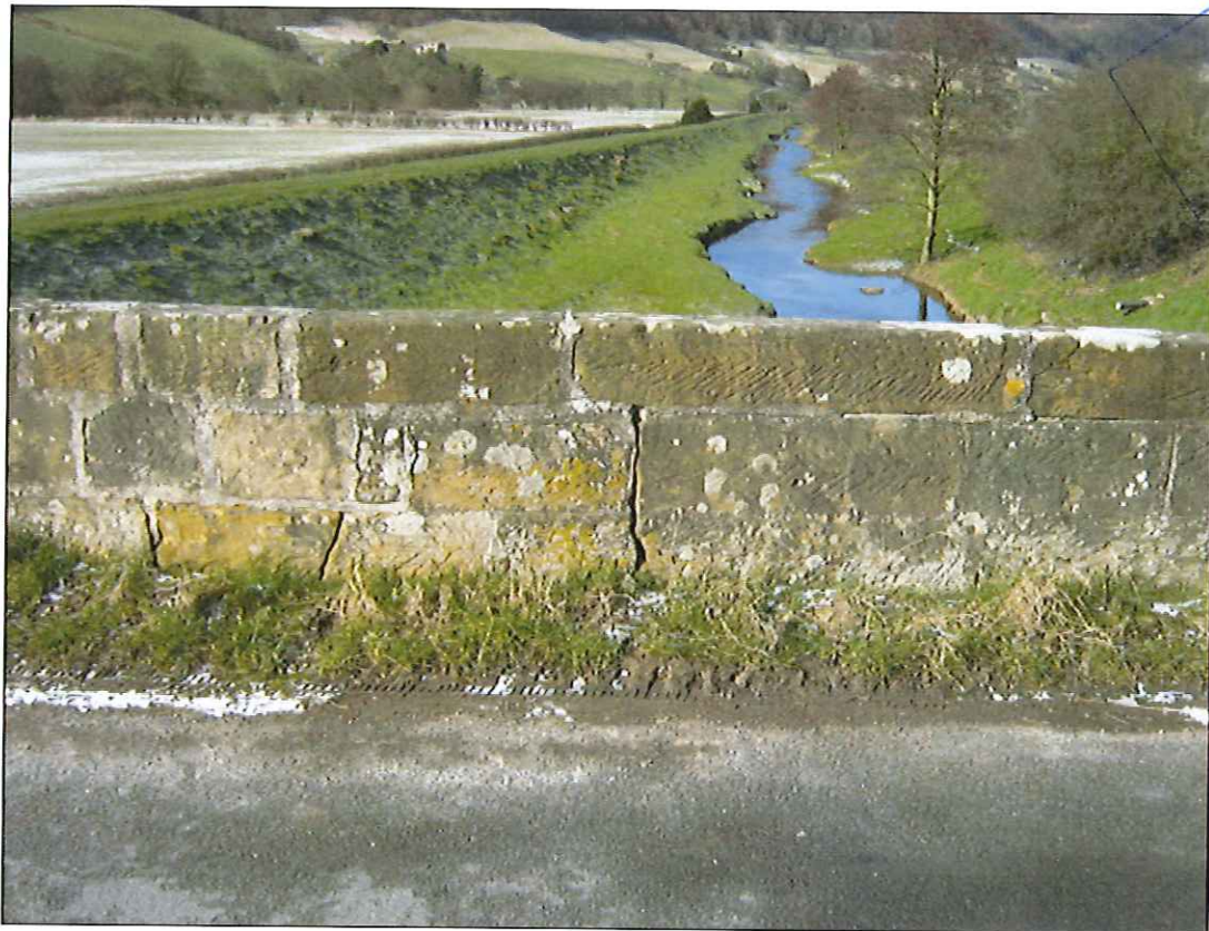
Photograph 41: Cracking to inside face of western upstream parapet, possibly due to vertical joints not being staggered.
