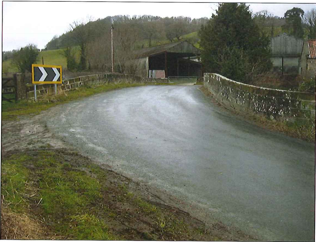
Photograph 2: View across bridge from south. Note narrowing carriageway width between parapets at centre of bridge.
