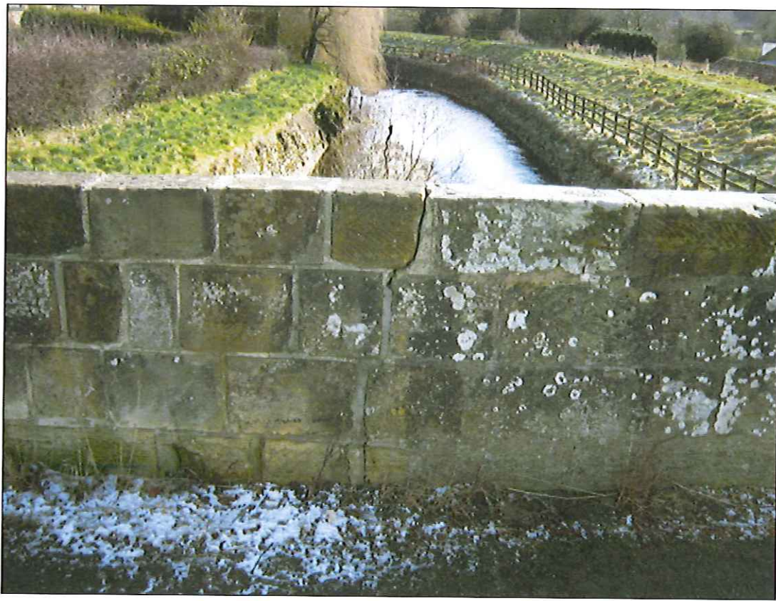
Photograph 42: Cracking to inside face of eastern downstream parapet. Note poor arrangement of vertical joints in stonework.
