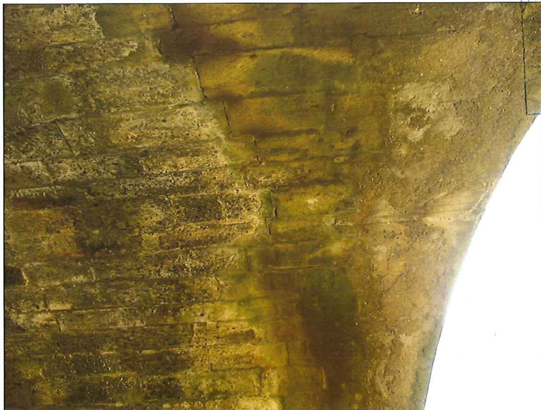
Photograph 32: Concrete widening #4 to western upstream side of north span. Note circumferential cracking in masonry further into arch.
