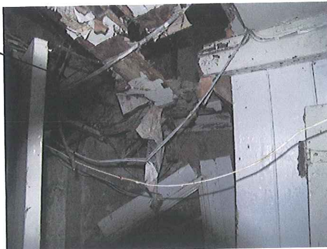
Collapsed first floor landing:
