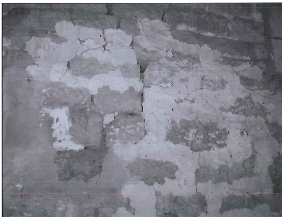
Figure 14: Crevices in internal walls
