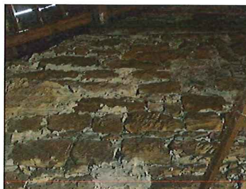
Photo 6: Internal crevices in garage
