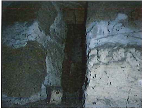
Photo 7: Large internal crevice
