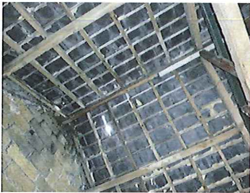
Photo 3: Internal ridge of garage is clear in places but not polished
