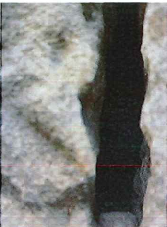
Photo 11: Cobwebs and mouse droppings found within large crevice in west wall
