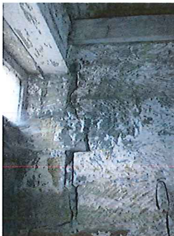
Photo 12: Large internal crevice
