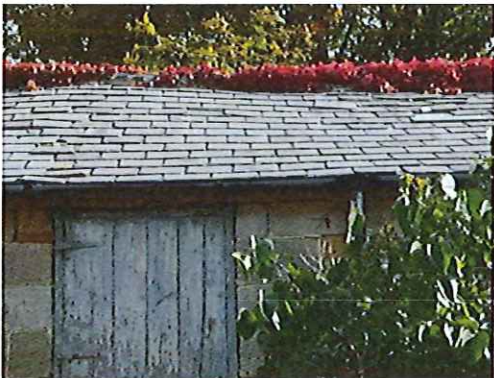
Photo 9: Slipped tiles west side of roof
