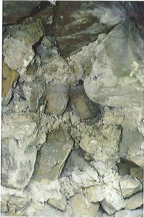
Photo 11: Collapsed area of wall
