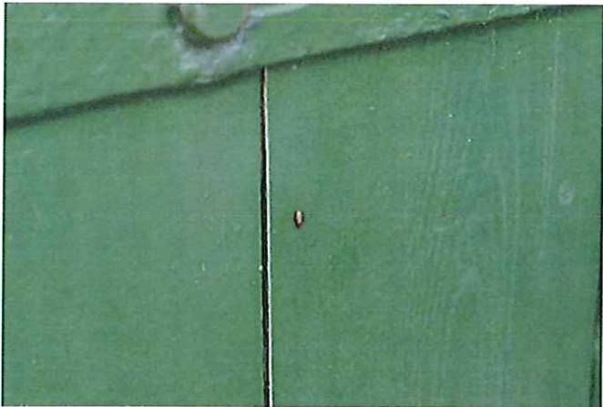
Photo 29: Bat Dropping on door 2
