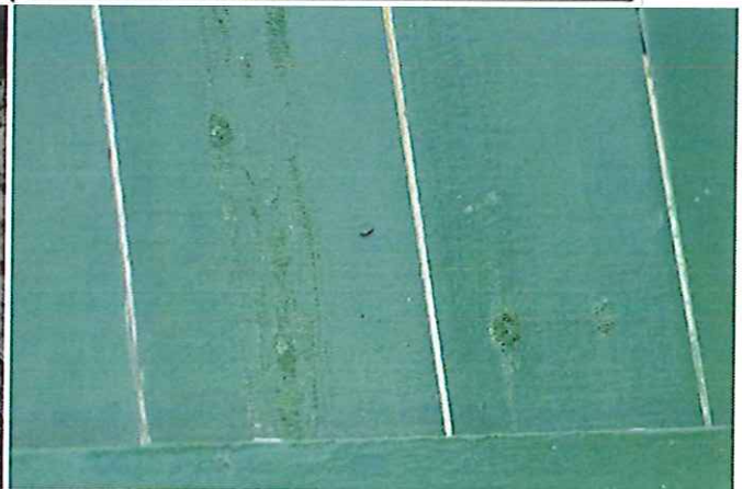
Photo 28: Bat dropping on door 1
