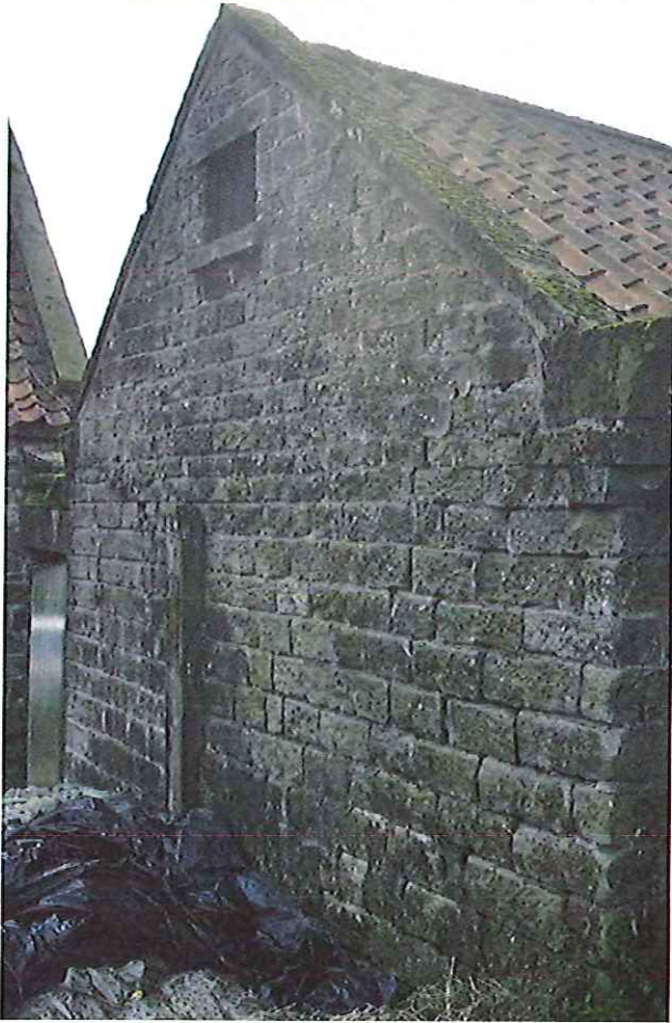
Photo 10: Poor condition of gable end wall
