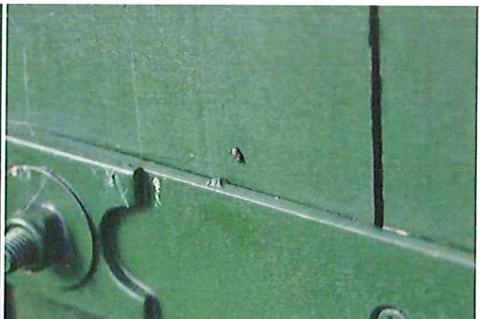
Photo 30: Bat dropping on door 3
