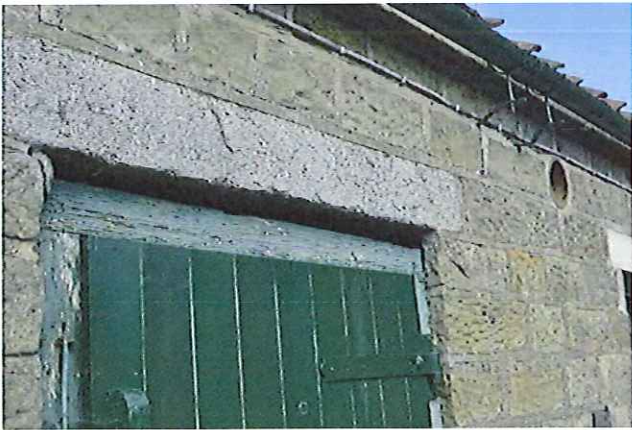
Photo 6: Gaps above doorframe
