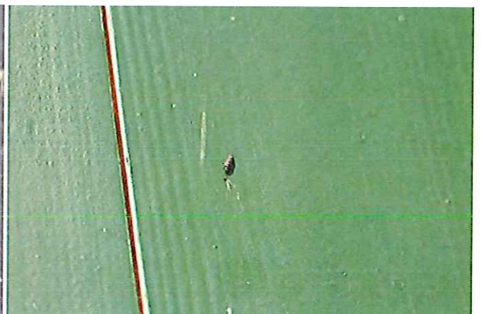
Photo 32: Bat dropping on door 4.
