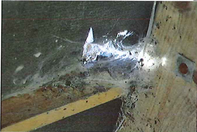
Photo 17: Hole in sarking
