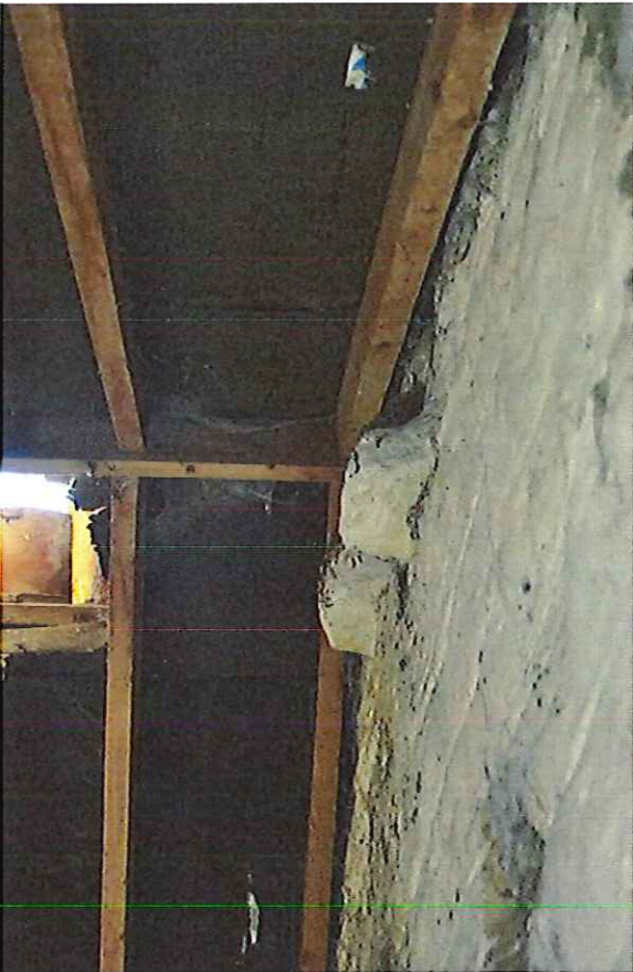
Photo 25: Gaps between rafter and gable end wall.
